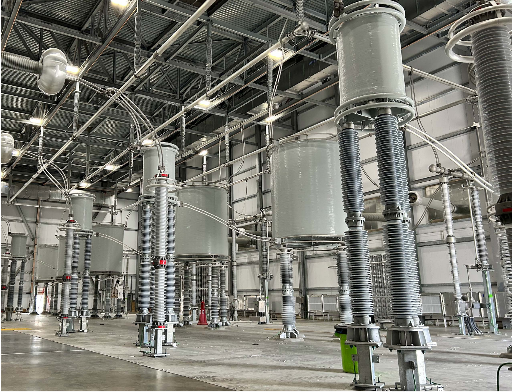
Inside the Astoria Converter Station's reactor hall, reactors stabilize the power after it has been converted from direct current to alternating current in the adjacent valve hall.
