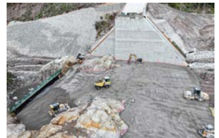
Crew members place roller-compacted concrete for the left abutment of the Cheekye Debris Flow Barrier.
